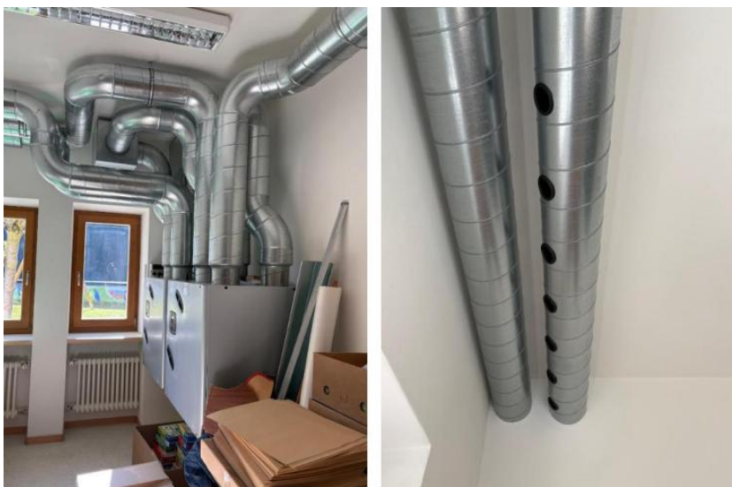
Fig. 4. VMC system installed in the office building. In the photo on the right: distribution system.
