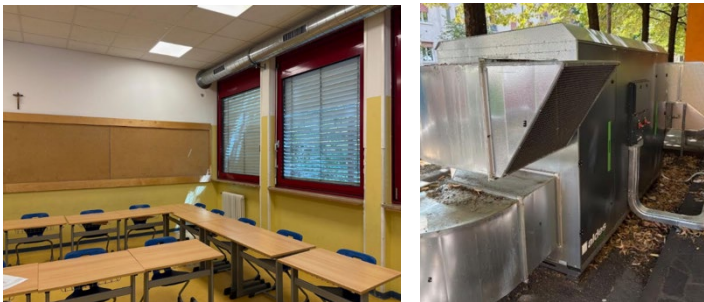
Figure 2. Distribution system in the classroom (left) and VMC installed outside (right). The machine serves four classrooms and a canteen. Primary school in Bolzano.
