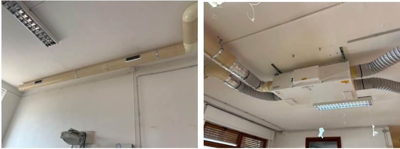
Figure 4. Distribution system in the classroom (left) and VMC installed in the corridor (right). One machine dedicated to each classroom. Secondary school in Bari.
