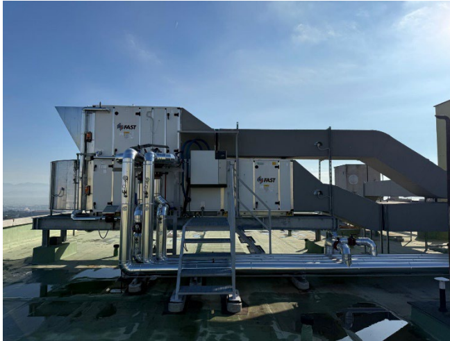
Figure 3 – The AHU rooftop of the UTIC section
