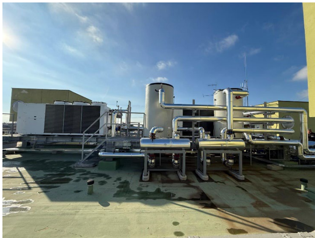
Figure 2 – The rooftop heat pumps of the UTIC section
