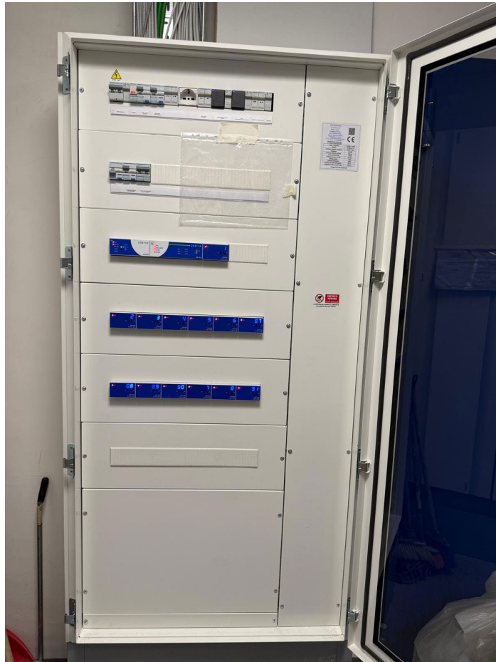
Figure 9 – Physical view of the electrical panel with controllers and expansions
