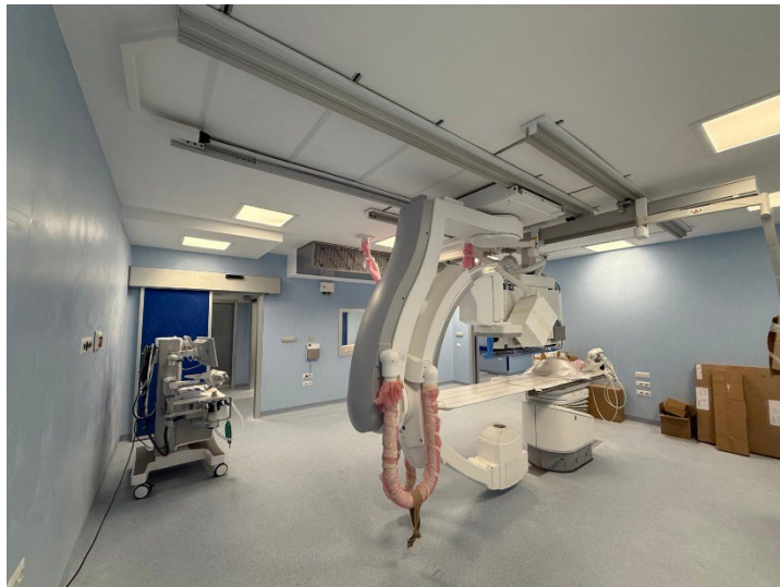
Figure 4 – One of the ICU rooms, in the background there is a VAV box
