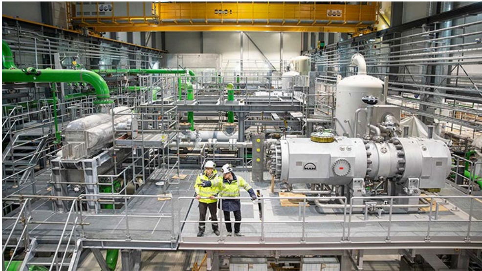
Fig 1. Example image, not exhaustive, just for illustrative purpose of MAN Industrial Heat Pump installed in the modern heat pump hall near the Esbjerg Harbor (Denmark) [4] which houses the world's largest seawater (Renewable Energy Source according to RED Directive) heat pump, which replace coal-fired heat plant for district heating application. Electricity for the heat pumps is generated by giant offshore wind farms producing an abundance of clean energy, making the district heating 100% based on renewable energy.
