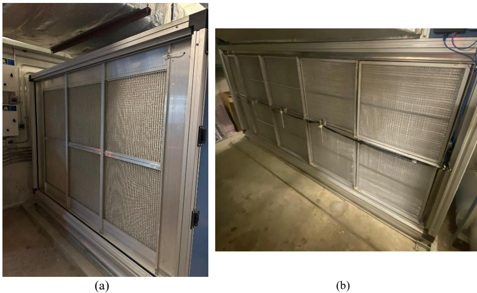
Fig. 1 Air filters in the AHUs' filter section for (a) AHUs in Building #1, and (b) AHU in Building #2. The first layer of washable metal prefilters can be seen.
