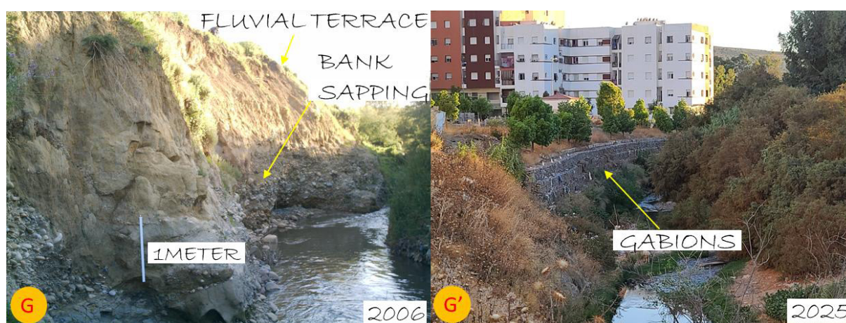
Fig. 12. Riverbank stabilization at section G. (G) Active bank erosion, 2006. (G') Gabion-reinforced bank with residential.
