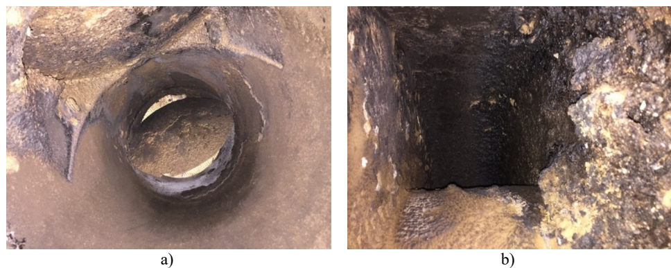
Fig. 2. Existing round suction ductwork with the control damper (a). Existing rectangular exhaust ductwork after the suction fan (b).
